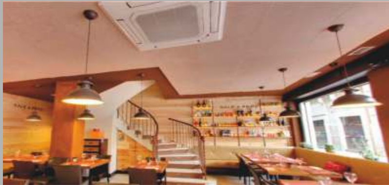
Acoustic Panels on ceiling.
